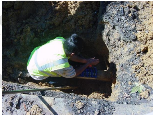
Figure 1. A member of Town crew works to repair a water leak on South Main Street (photo by Town staff).
